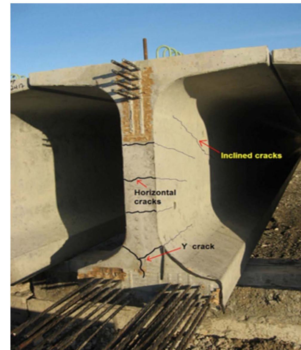
Figure 2. Inclined and Horizontal End Cracking on Girder (Photograph by Concrete Bridge Views)
